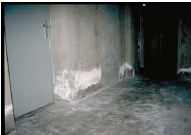
Figure 3.3 : Efflorescences (EPQR Rénovation).
